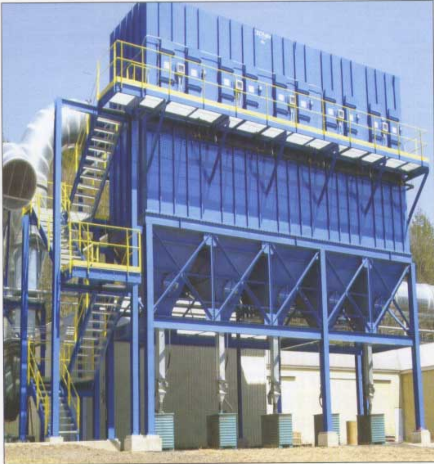
North dust collector powered by a Baldor Super E 200 hp electric motor
