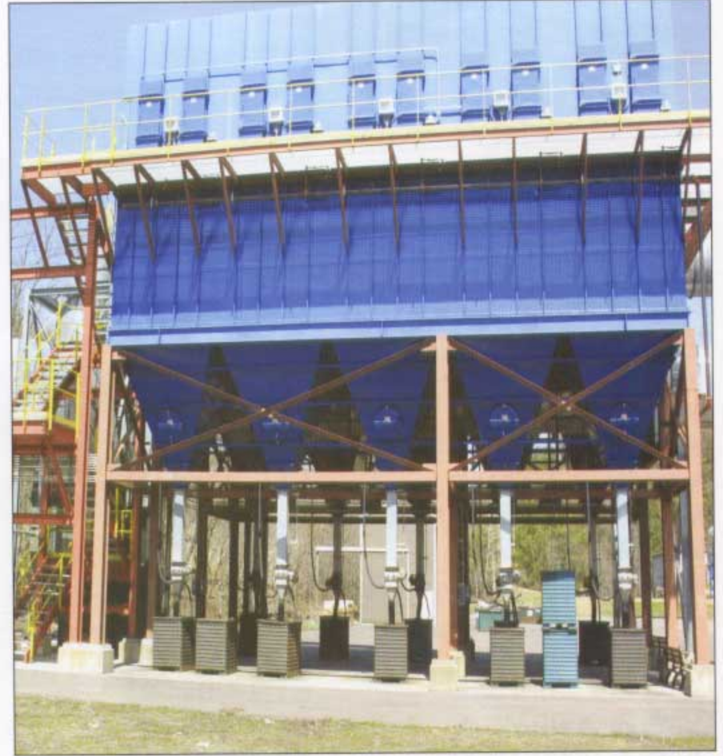
South dust collector powered by a Baldor Super E 500hp electric motor.
