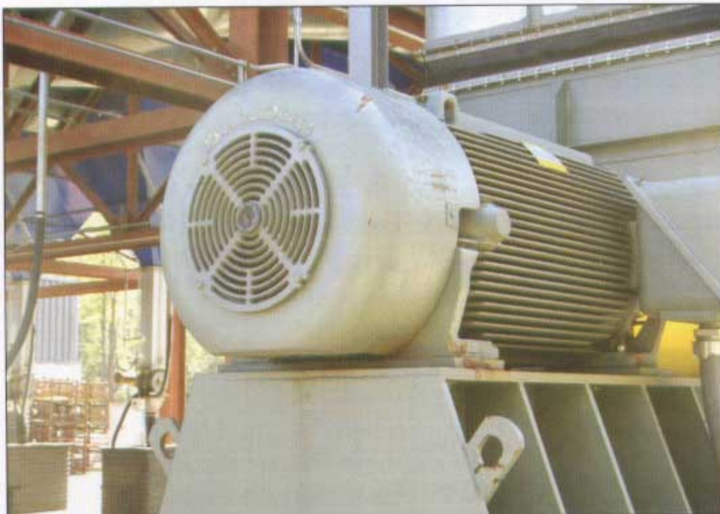
Close-up of the Baldor Super E 500hp electric motor.
